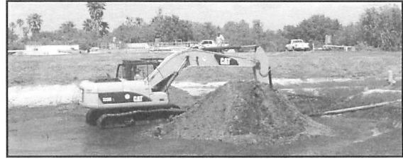
The District is attempting to create what is known as Perk Ponds at the existing plant site.
