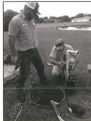
STEP system Repair SLID has taken over operation and repair of Waste Water STEP system
