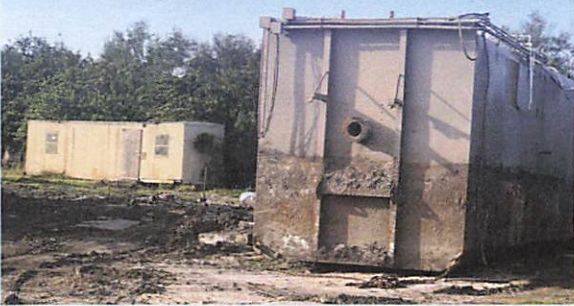
The site of the former sewer plant is close to being fully demolished as the storage tanks are the only thing left.
