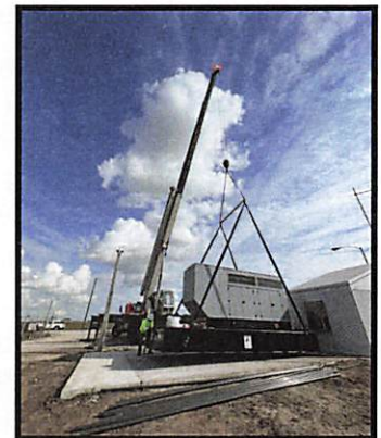
Generator being installed at Water Plant #2 as part of the renovation and upgrading project. This back up plant is located on the west side of the District on the site of the former power plant.
